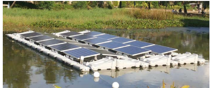
A solar pilot project on a flood control waste pond in Indonesia. Credit: Ciel & Terre International
